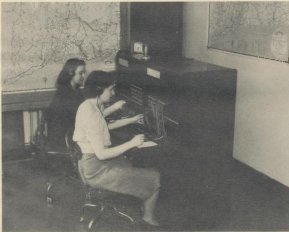
Telephone switchboards, recently installed for all department lines at Hartford, provide constant service to the public. The Misses Helen and Clairann Noonan, sister operators, are fully informed of the multitudinous services of the various department offices and divisions.
